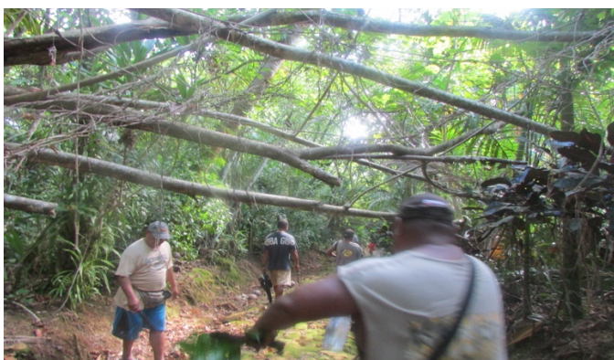
Photo Courtesy of TRCT: Community Members in Maa, Tamil, undertaking preparation work at the designated project site
